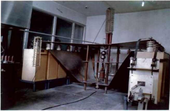
High Current Generator, 48.6 kJ Pre conditioning at 100kA before OD Test
