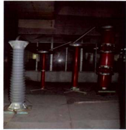
Partial discharge test on 168kV Arrester with 300kV Test Transformer
